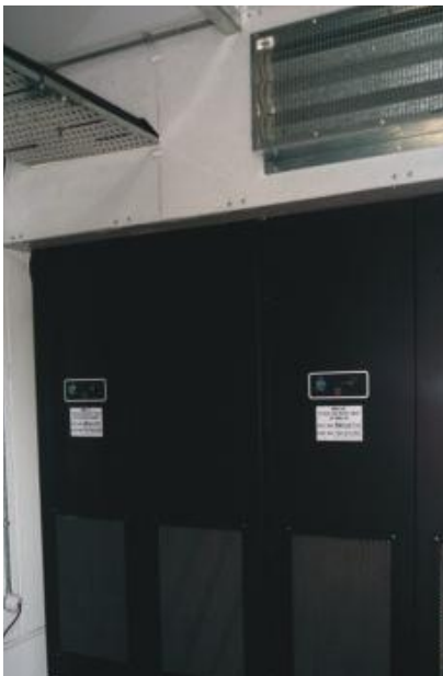
Example CleanSource® UPS
